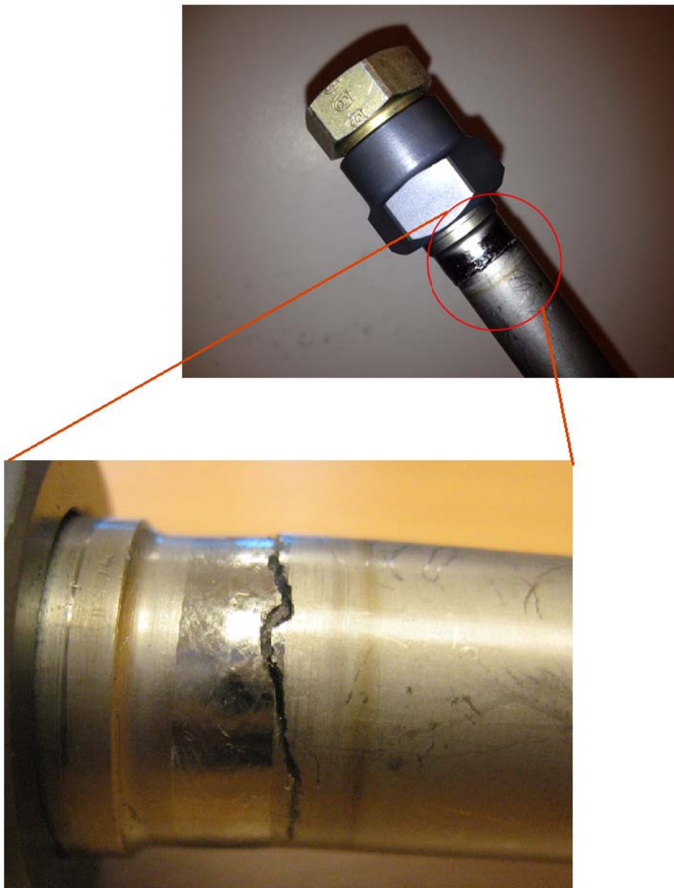
Figure 10: Cracked hydraulic tube
